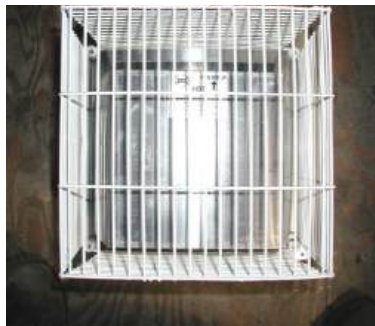
VIEW OF SAFETY CAGE
