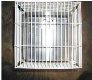
VIEW OF SAFETY CAGE
